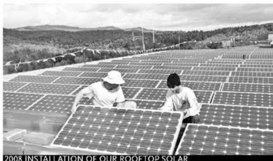
2008 INSTALLATION OF OUR ROOF TOP SOLAR
